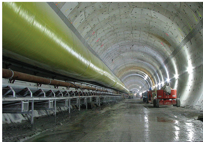
Clem Jones Tunnel — Brisbane
